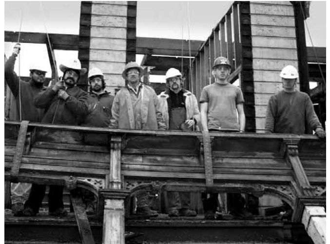
Workers with the ReBuilding Center of Portland, Ore., "deconstruct" a house, meaning that they take it apart in the reverse order that it was built. The center will then resell the materials.
